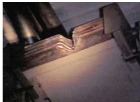
Burned “V” Shape in Bus Bar Plates
