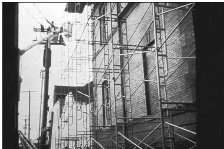
This power company worker is placing insulated sleeves ("eels") over the power line in this photo.
