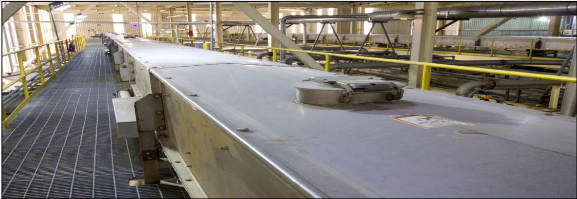
Figure III. 3. Enclosed Belt Conveyor
