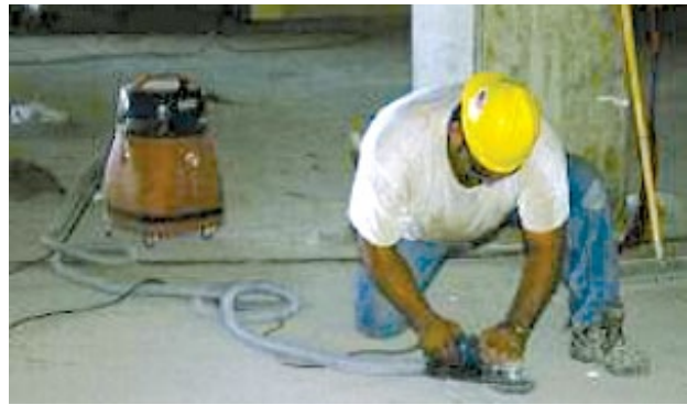
A worker using a grinder with an attached vacuum dust collection system. The vacuum pulls dust through the hose, where it is captured by filters. (Photo courtesy of the University of Washington)
