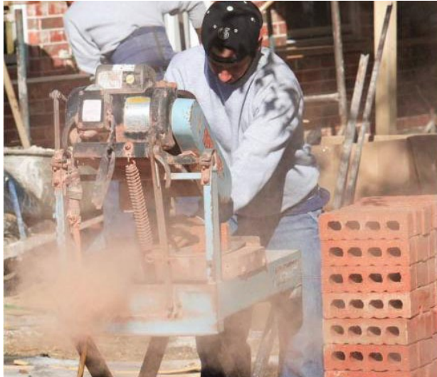
Using a stationary masonry saw without dust controls can expose workers to high levels of silica. Table 1 provides a simple explanation of what employers can do to keep their workers safe. (Photo courtesy of CPWR)
