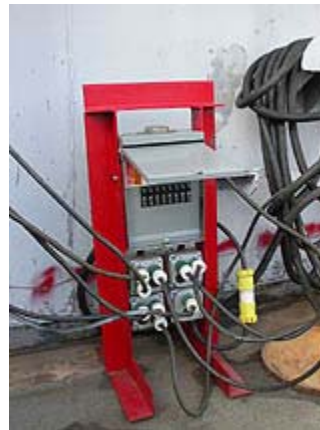
Circuit breakers in panel box can be used to deenergize circuits (and appropriately tagged) before working on the circuit.
