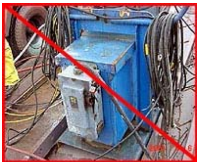
Improper practice - Faulty breaker box presents shock hazard.
