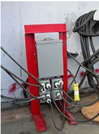
Portable distribution panel used to supply temporary electrical power.
