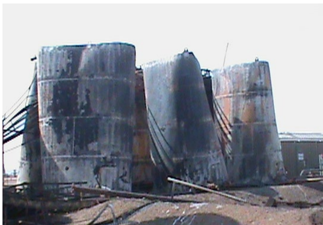
Figure 2: Damaged storage tanks from flare flashback event.
