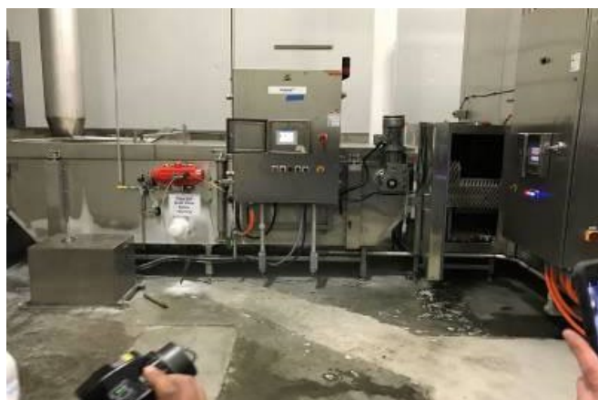
Figure 1: Six workers died from a low oxygen atmosphere when nitrogen was released from flash freezing equipment.
