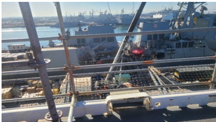
Image shows use of a guardrail at the deck's edge to prevent workers from falling to a lower level.
