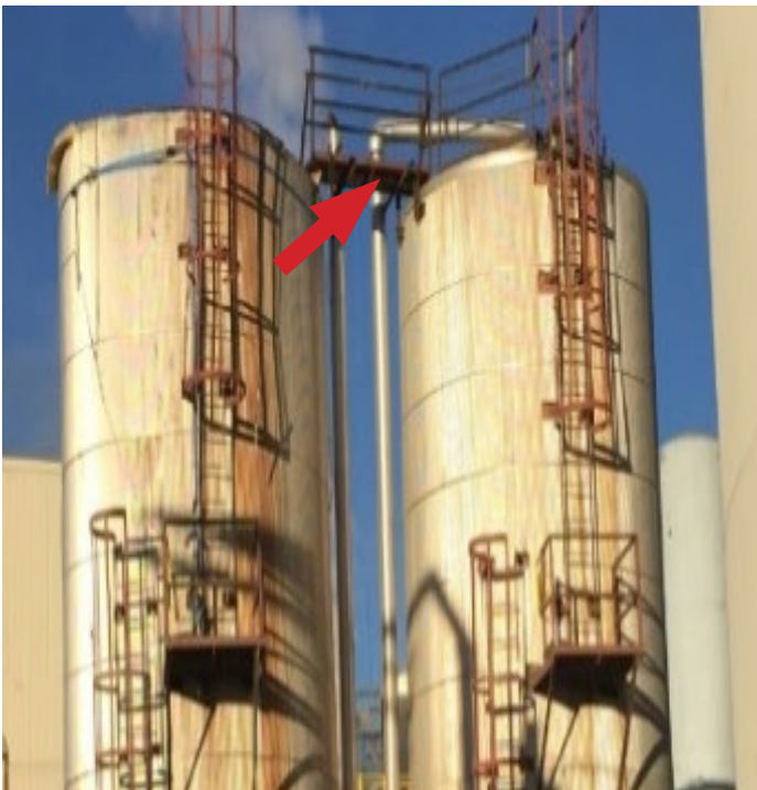
Figure 1: Soapstock tanks (red arrow shows where worker was welding when tank on left exploded).
