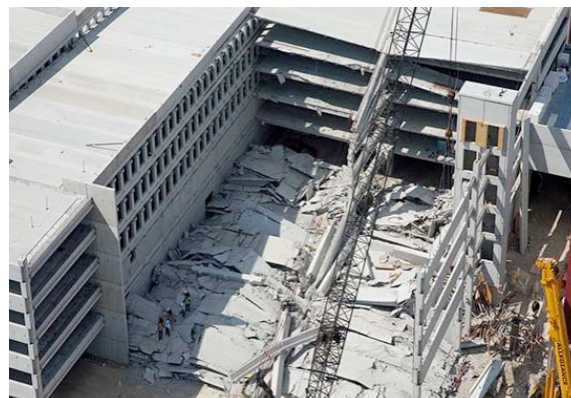
Figure 1: Aerial view of collapsed garage
