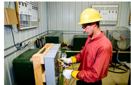
Worker testing the wiring on equipment to ensure the equipment is deenergized
