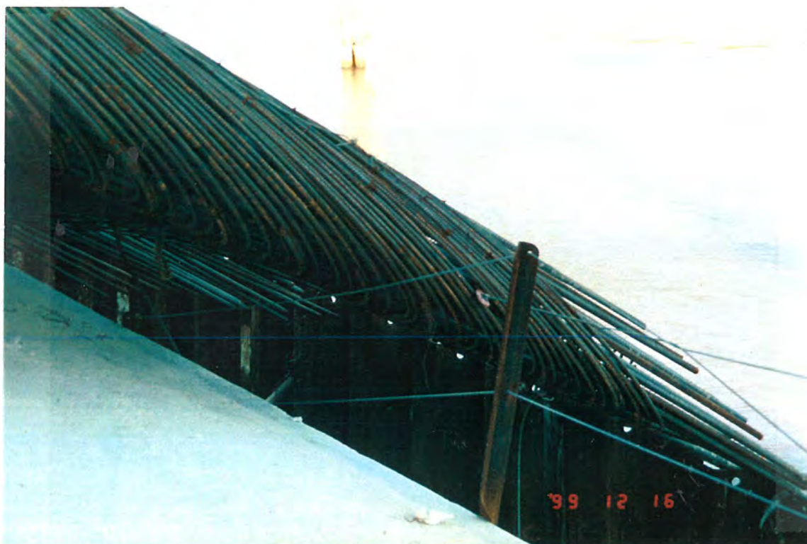
Figure 3-10 The Upper Free End of the Collapsed Steel Cage (Looking toward North from the Concrete Footing).
