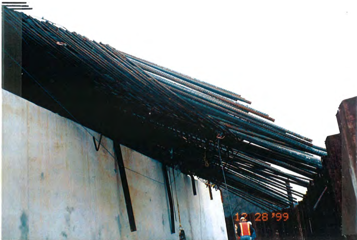
Figure 3-11 The Upper Free End of the Collapsed Steel Cage (Looking upward from the Alley between the Side of the Concrete Footing and the Steel Sheet Piling).
