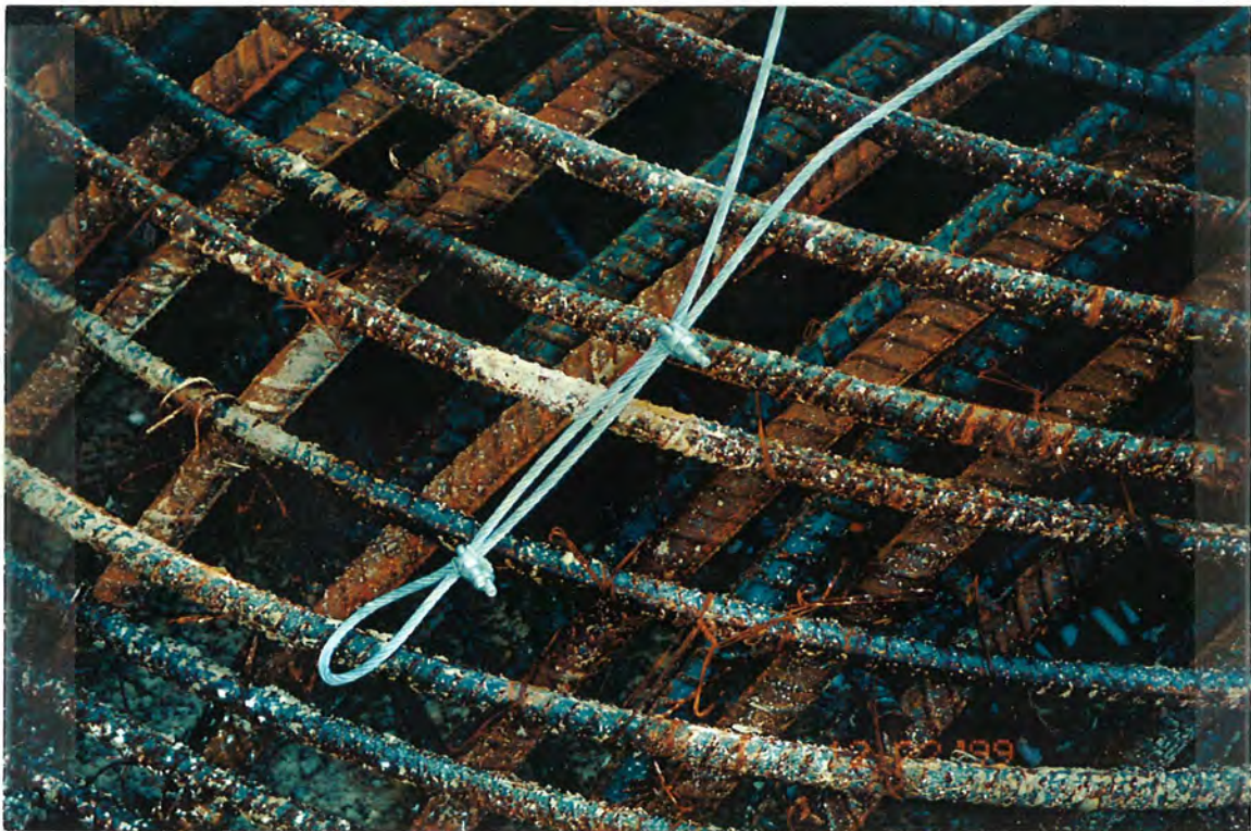
Figure 3-20 The Lower End of the Southwest Guy Wire. Please note that there were no damages observed on this end of the wire.
