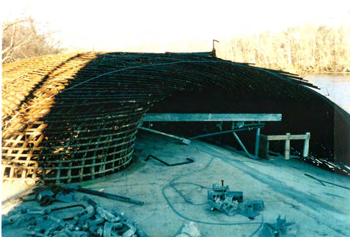
Figure 3-7 The Bottom Fixed End of the Collapsed Steel Cage (Looking toward North from the Concrete Footing).
