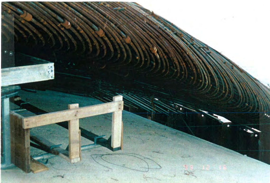
Figure 3-9 The Middle Portion of the Collapsed Steel Cage (Looking toward North from the Concrete Footing).
