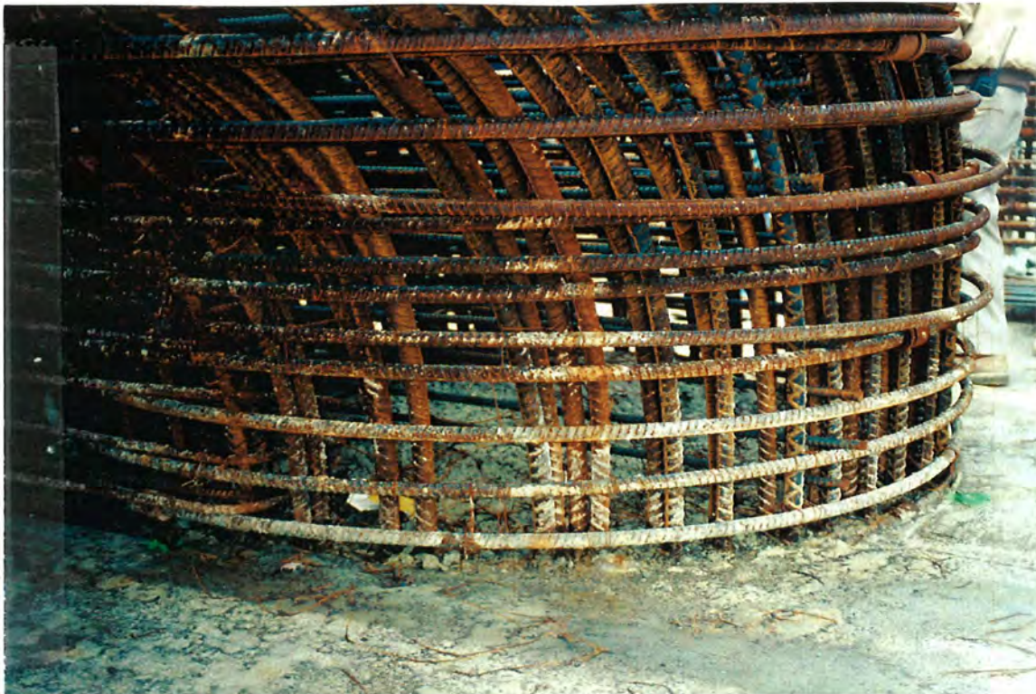
Figure 3-15 The Condition of the Collapsed Steel Cage at its North Fixed End (Looking from the Concrete Footing).
