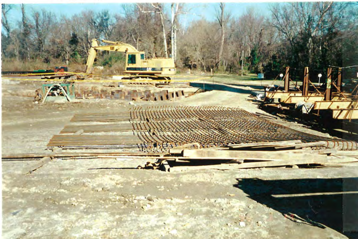
Figure 3-16 The Last Section of West Face Extension Did Not Install to the Collapsed Steel Cage.
