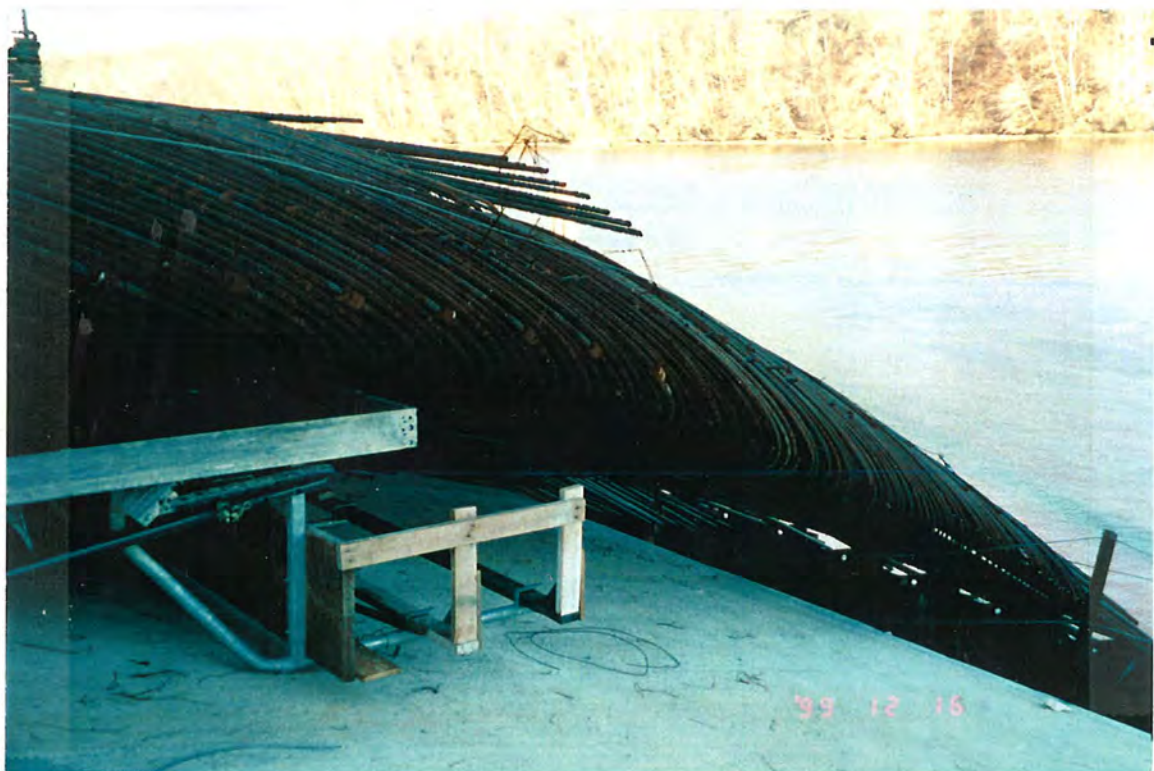
Figure 3-8 The Lower Portion of the Collapsed Steel Cage (Looking toward North from the Concrete Footing).
