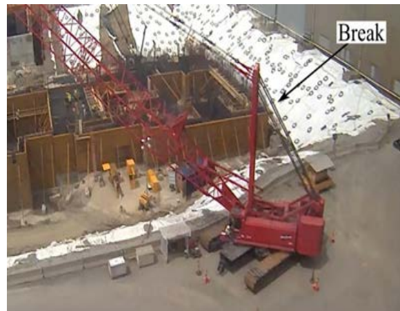
Photo 3: Wire rope failure location in the lattice boom crawler crane.
