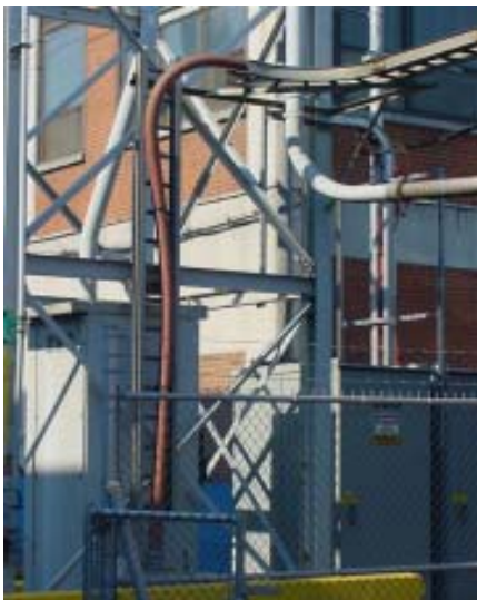
Figure 2. Outdoor metal clad cable in cable tray.
