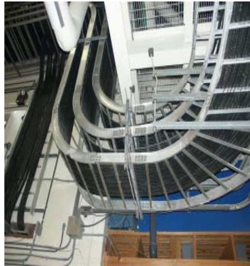
Figure 3. Electrical wires in multiple cable trays.
