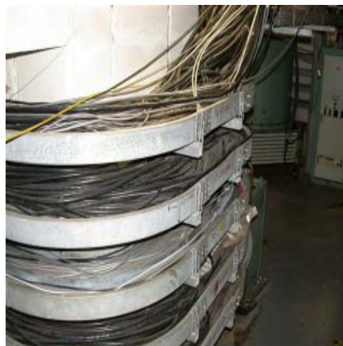
Figure 6. Overloaded Cable Tray.
