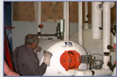
Fig. 2: Inspect all potential water sources.
