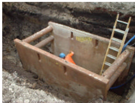
A trench box is being used—but what is wrong with this picture? Hint—what would happen if the soil on top collapsed?
