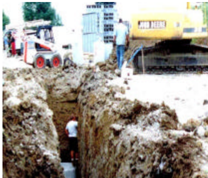
Luckily, this worker made it out of the trench alive.
