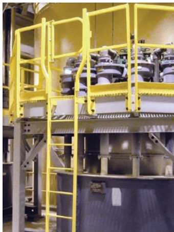
Raised platform with protected guardrail.
