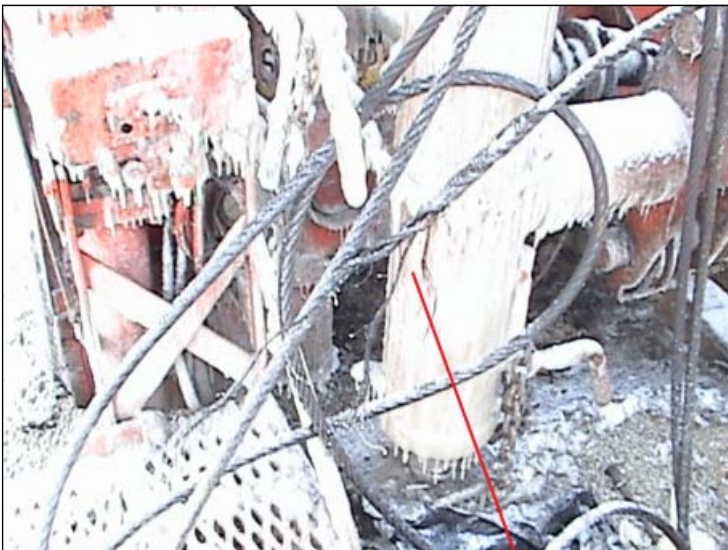
Location of failed 7/8" load line.
